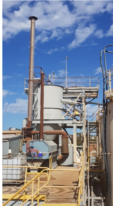
Furnace & Carbon Reactivation Kiln
